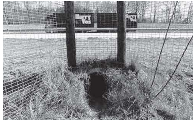
Picture 1 – Passage for small animals in the highway BR-101 south (Source: PBA – subprograma de proteção à fauna, 2001).
