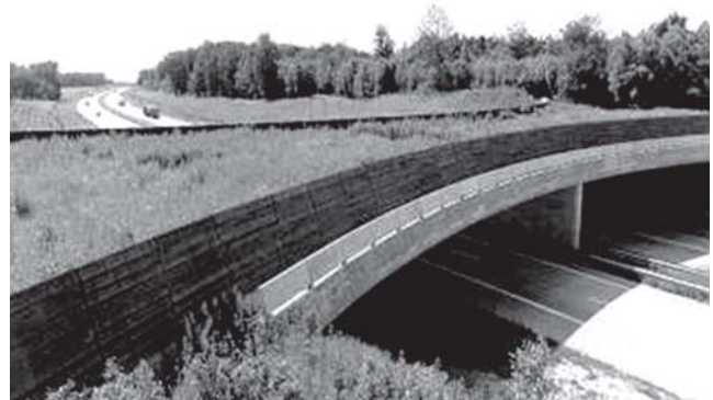
Picture 2 – Ecological bridge in the highway BR-101 south. (Source: PBA – subprograma de proteção à fauna, 2001).
